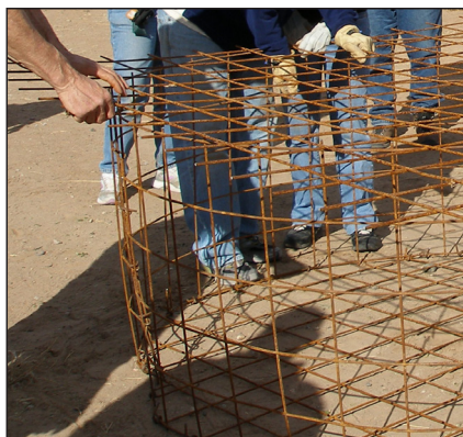
Constructing a beaver deceiver can be done in less than a day with a handful of volunteers.
